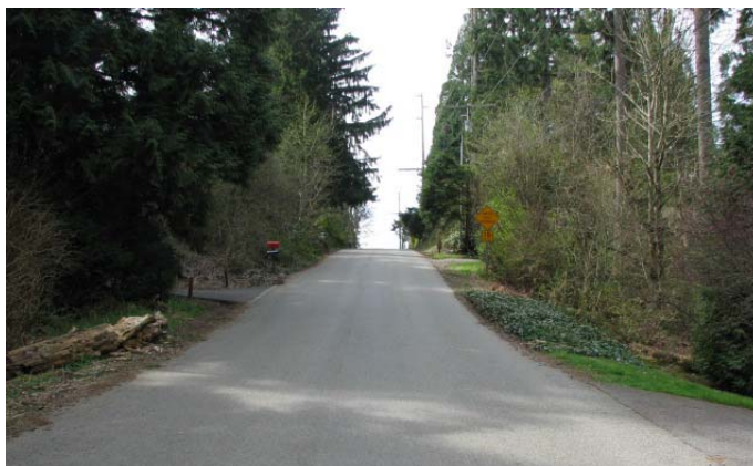
Photo 9: NE 195 th Street Approach Hill with Substandard Sight Distance
